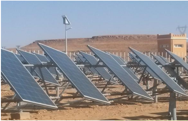
Fig. 1 1.1MW PV plant in Oued nechou (Ghardaia)
